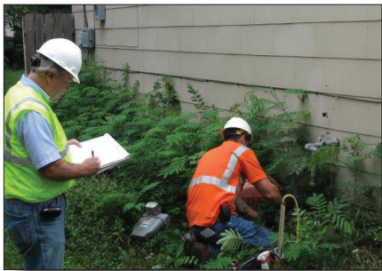
PSC Safety Engineering Staff member Greg Williams, left, inspects a gas line and meter installation.
