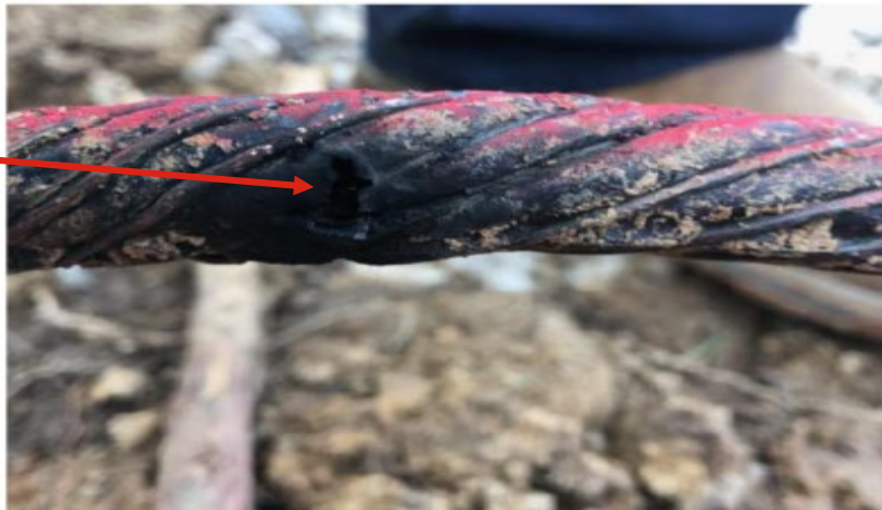
Faulted Direct buried #2 Al Cable with exposed concentric neutral
