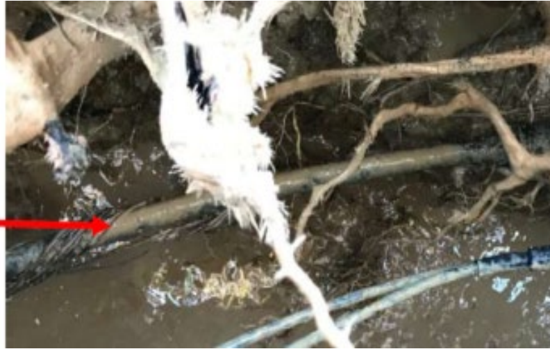
Exposed concentric neutral cable in ground with the neutral eroded away
